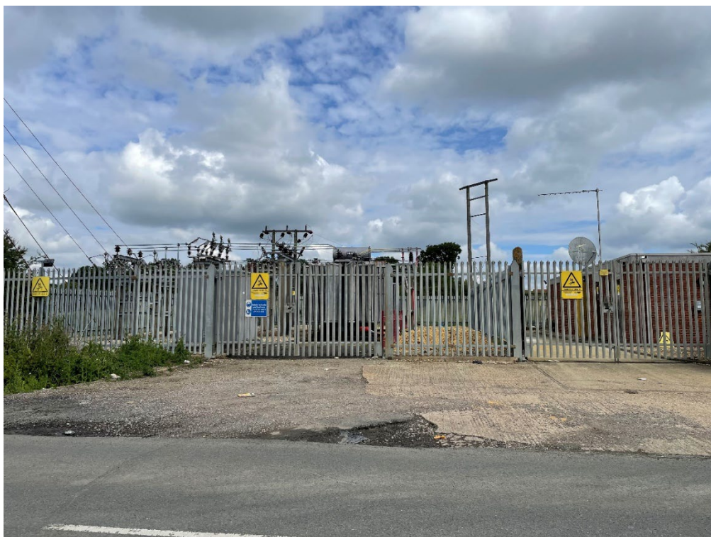
Plate 38 Electrical substation to the west of the site frontage
