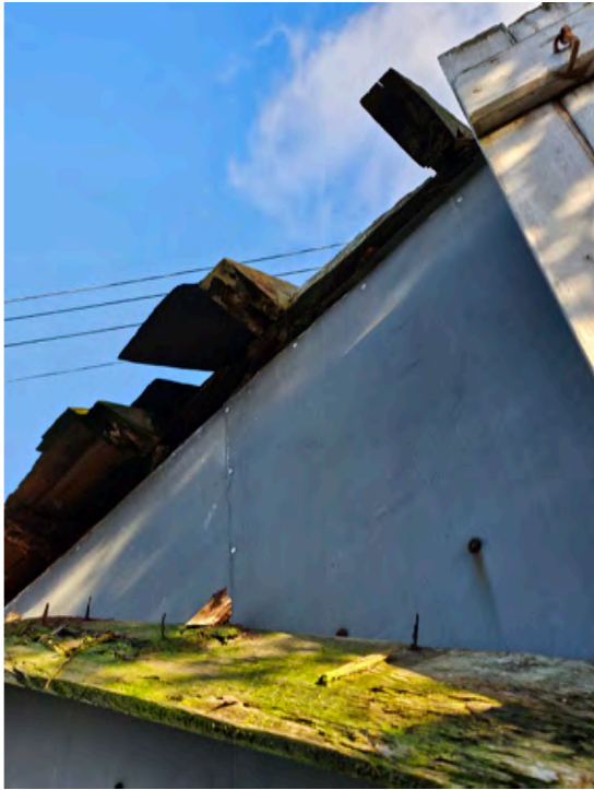
splayed rafter feet with nailed soffit board (displaced)
