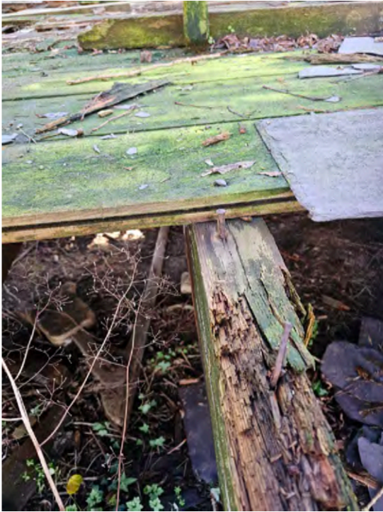
tongue and groove floorboards
