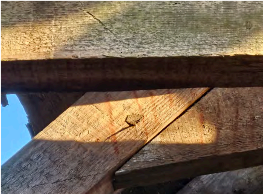
original pegged collar to rafter. Note red riddle pencil carpenter's marks rather than scribed with chisel suggestive of successive alteration to roof
