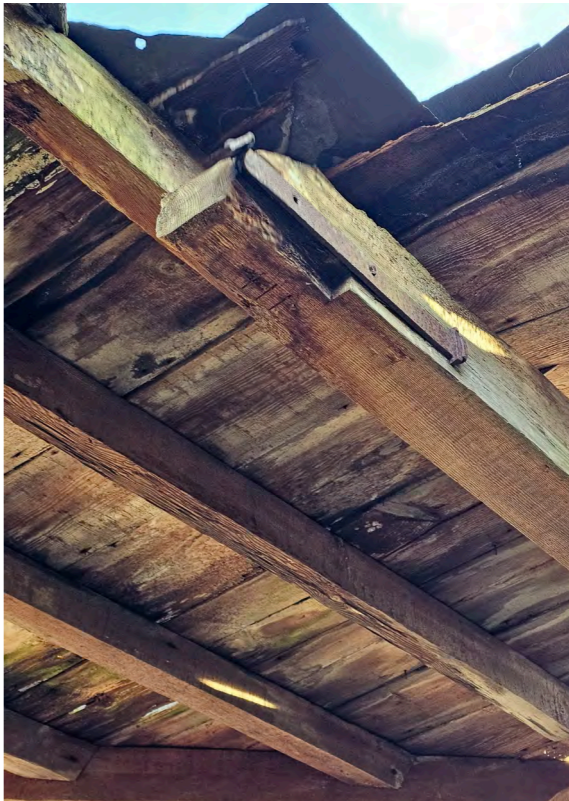
dovetail joint to tie beam to wall plate with twisted forged strap for restraint
