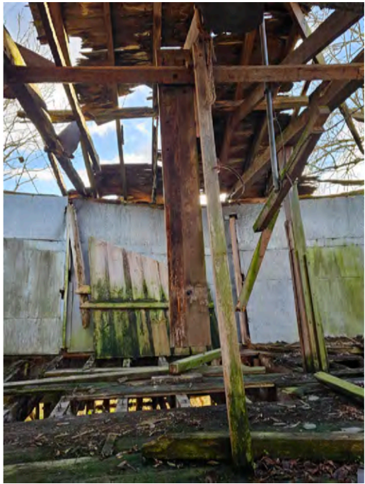
central grain bin prop supporting tie plate to be removed
