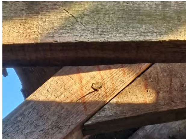
original pegged collar to rafter. Note red riddle pencil carpenter's marks rather than scribed with chisel suggestive of successive alteration to roof
