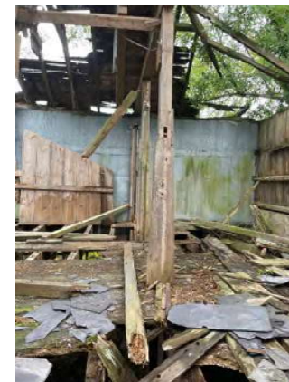
mortice and peg in grain bin post to receive partition and remnant of grain bin partition
