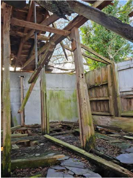
haunched and grooved central grain bin post supporting tie beam. NB brackets to be removed
