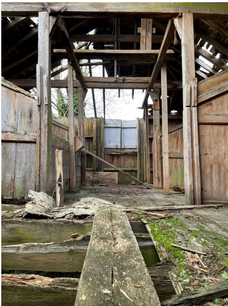
Plate 17: Structure A, detail of interior including missing and rotten floorboards and floor joists.
