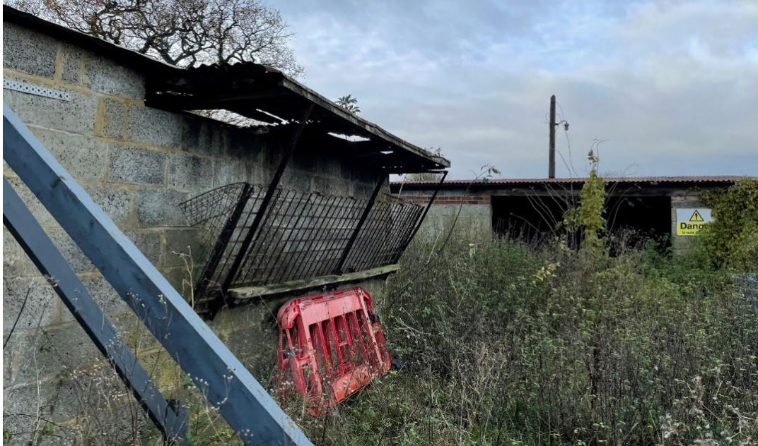
Plate 19: General view of Structures B and C looking south-west from adjacent to the north elevation of Structure B.
