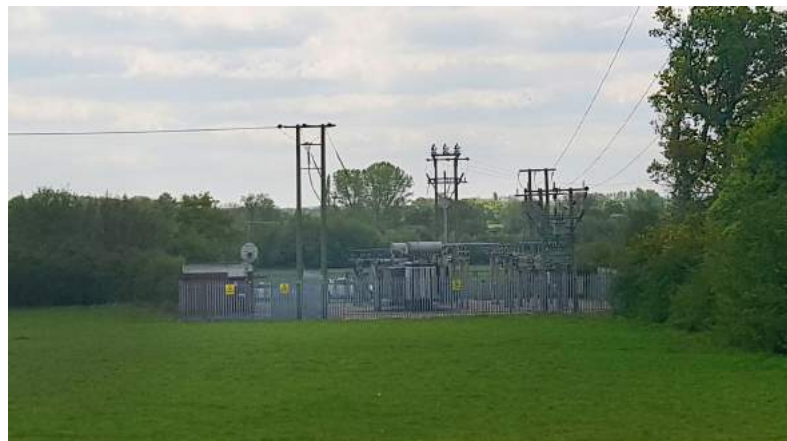
View south towards the electricity sub station
