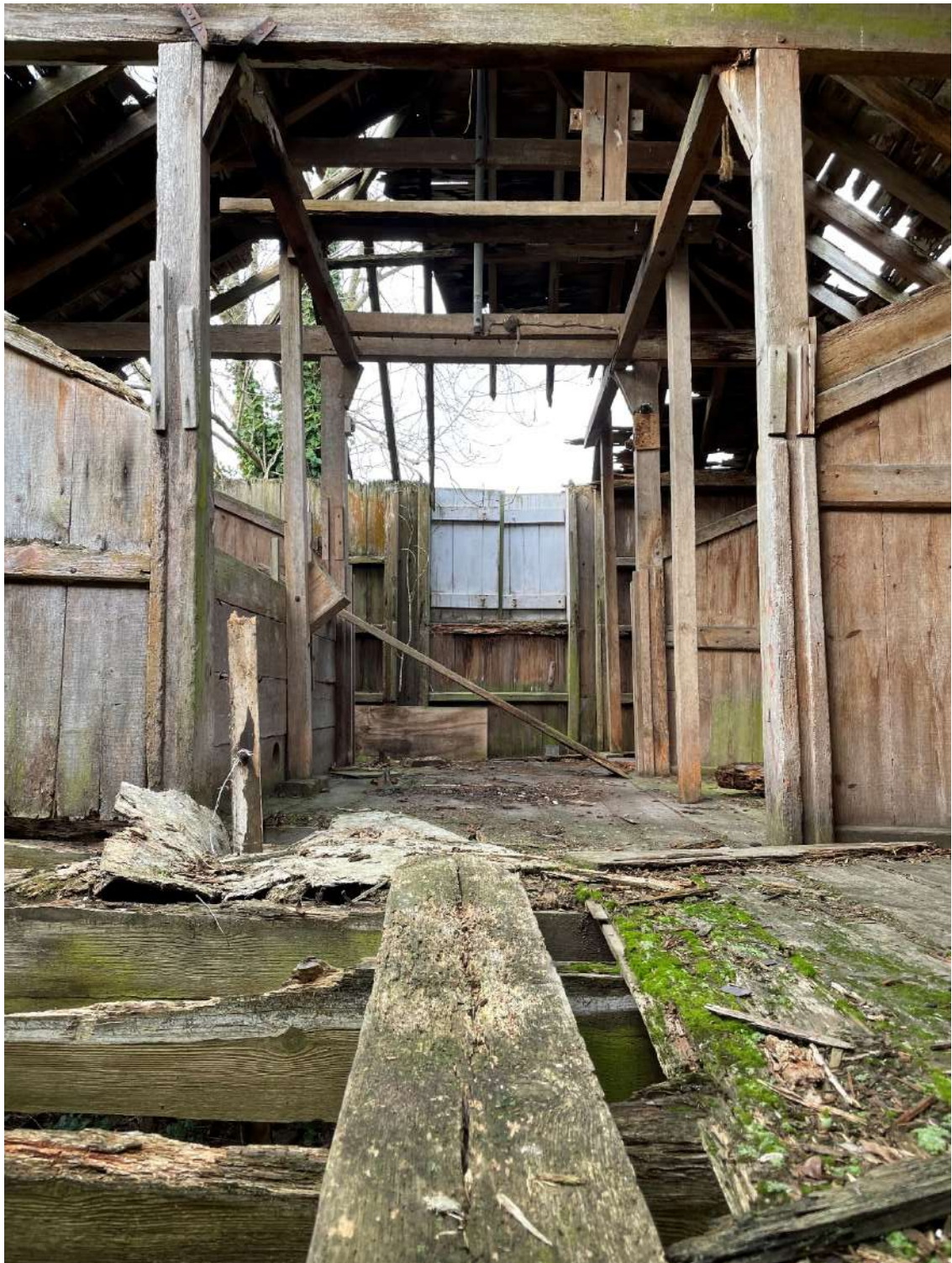
Plate 8: Structure A, detail of interior including missing and rotten floorboards and floor joists.
