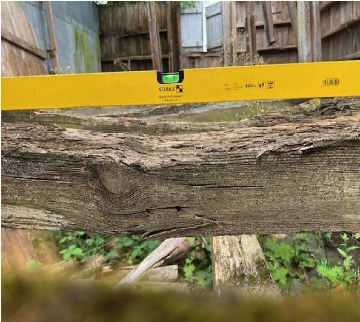
The level here shows that the timbers running W1 – W3 are fairly level, the decay through the timber where it has decayed and come away, details the misshape of the timbers.
