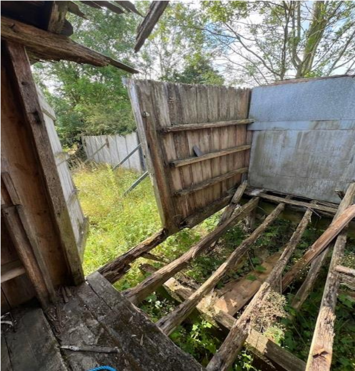
The main joists at W2 are in very poor condition, the rot is extensive throughout the full length of the timbers.
