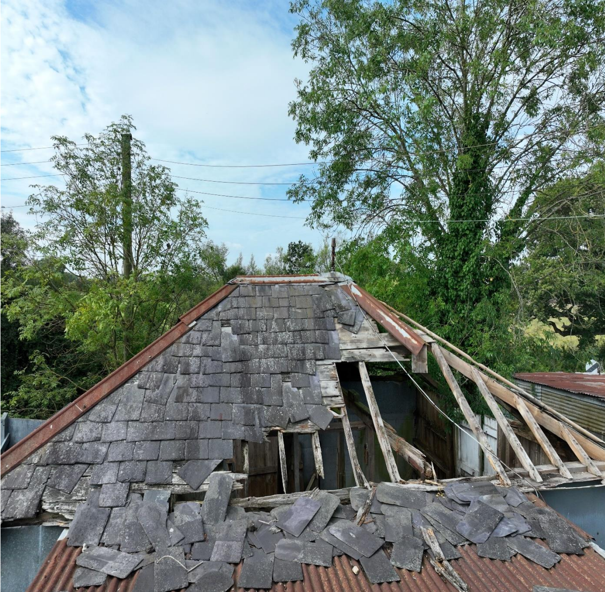
The drone photo here shows the extent of the decay of the roof.
