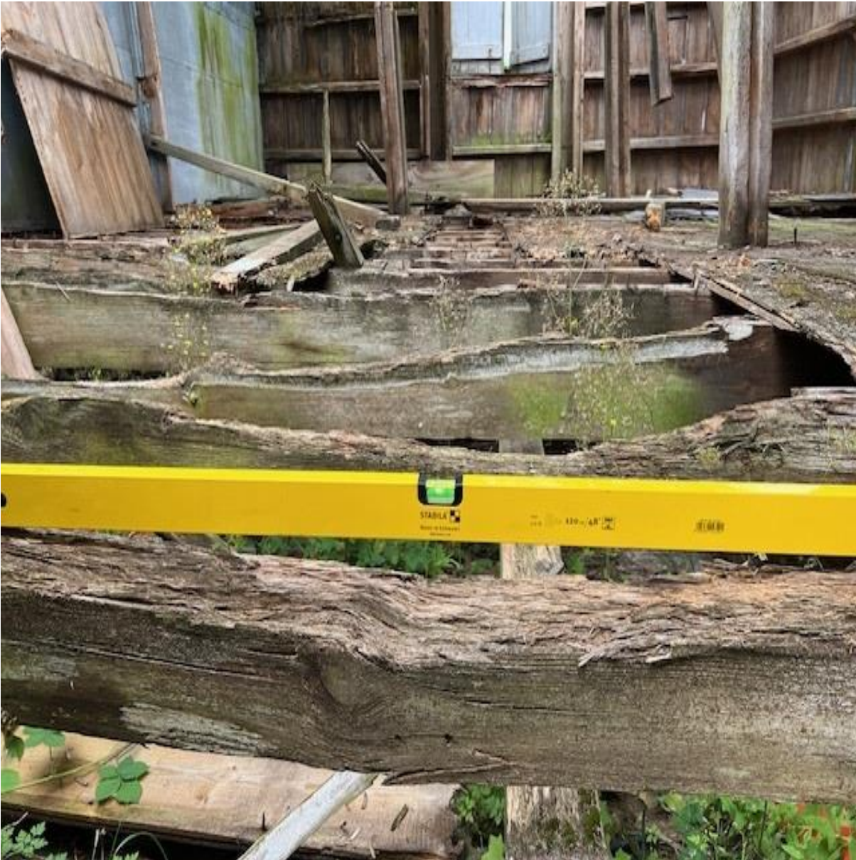
As above photo, it can be seen through the photo here the first 5 joists in particular extensively decayed.
