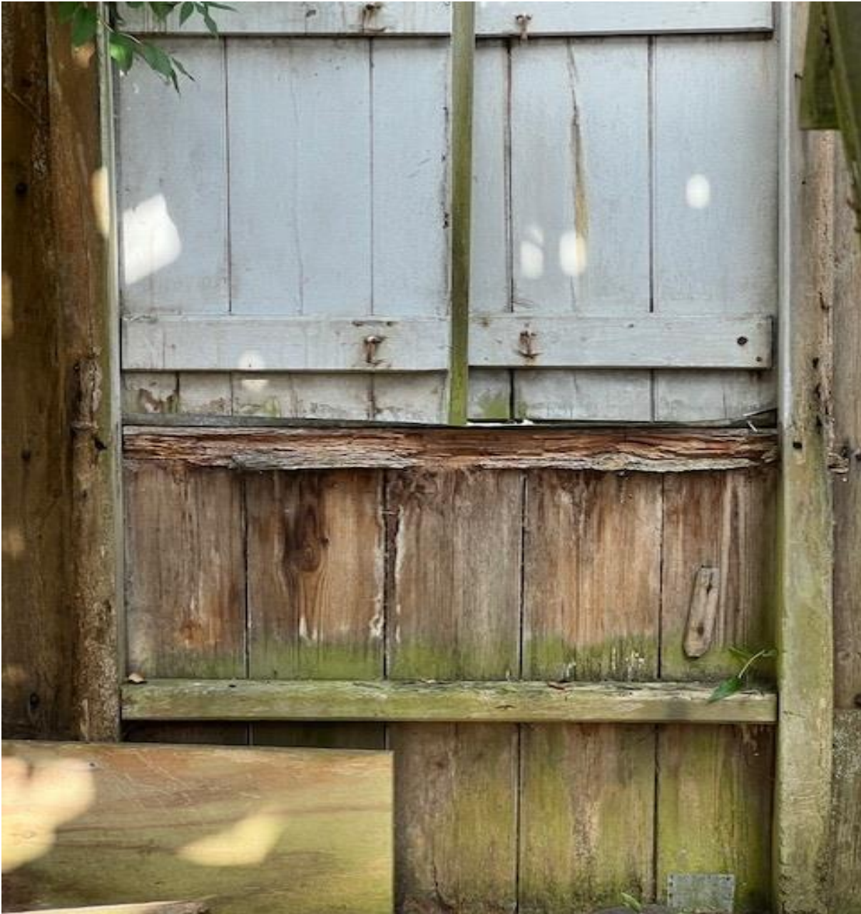
The timbers that sit under the shutter windows at W4 are decayed not only at the vertical timbers but also at the supporting horizontal timbers.
