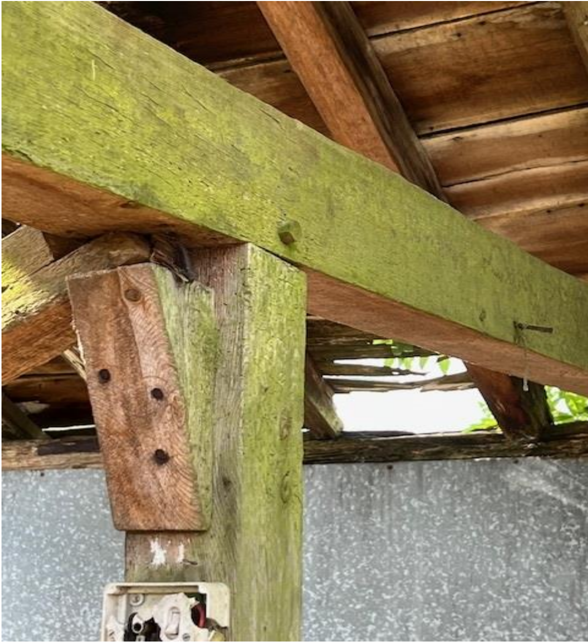
The cross timber here is also morticed at the head of another post, the other cross-sectional timber that sat over the ledge brace has now collapsed.
