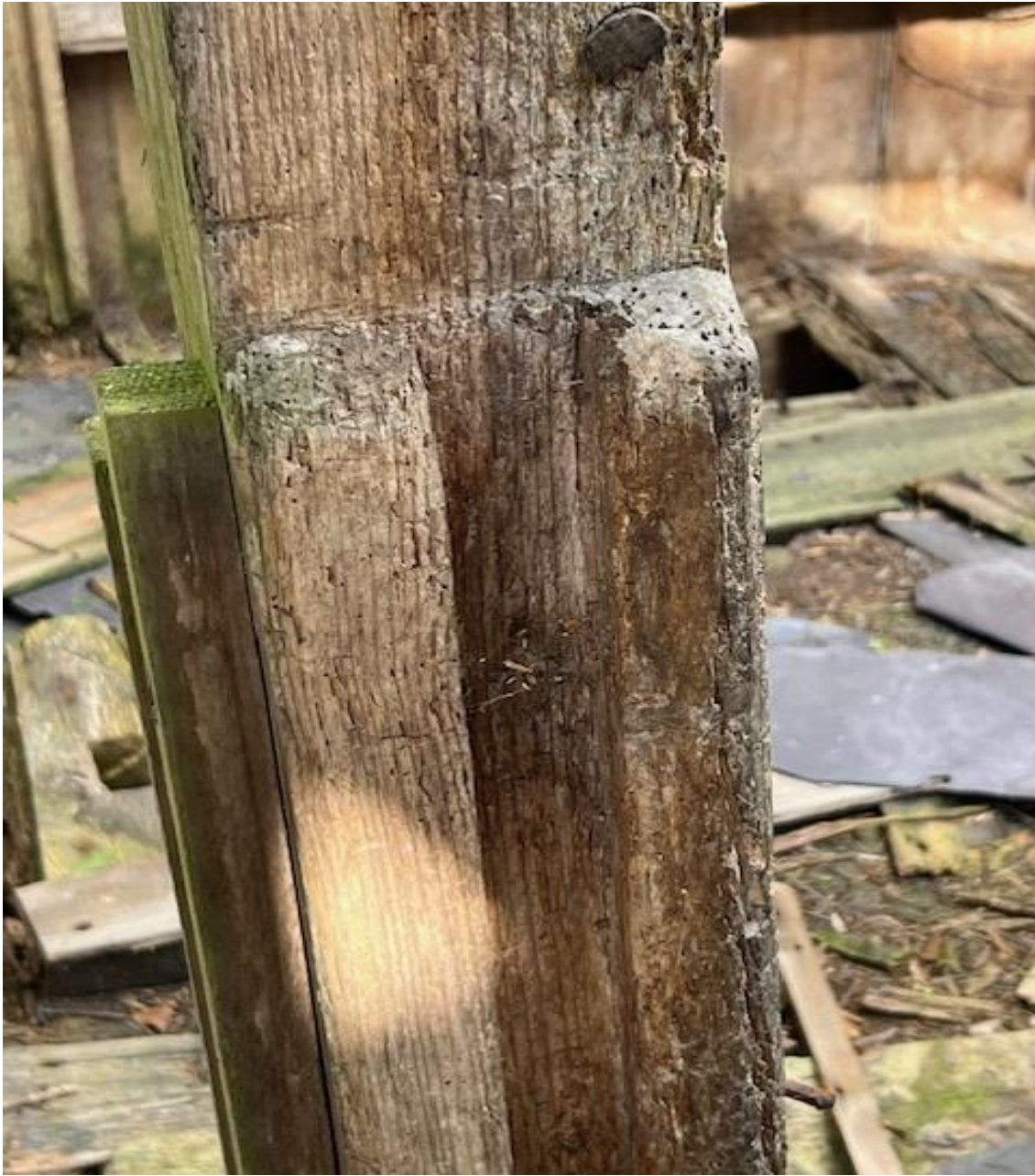
As above, the posts here are chamfered in style, but are now suffering from some slight wood boring insects and rot.
