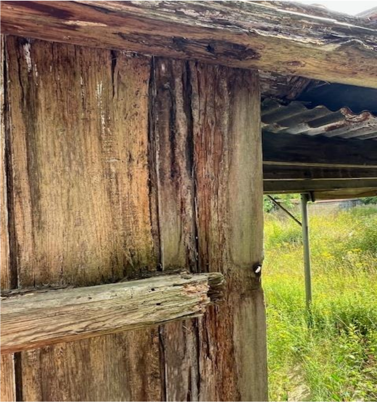
The vertical timbers at W1 show the timbers to be significantly decayed, as are the support horizontal timbers.
