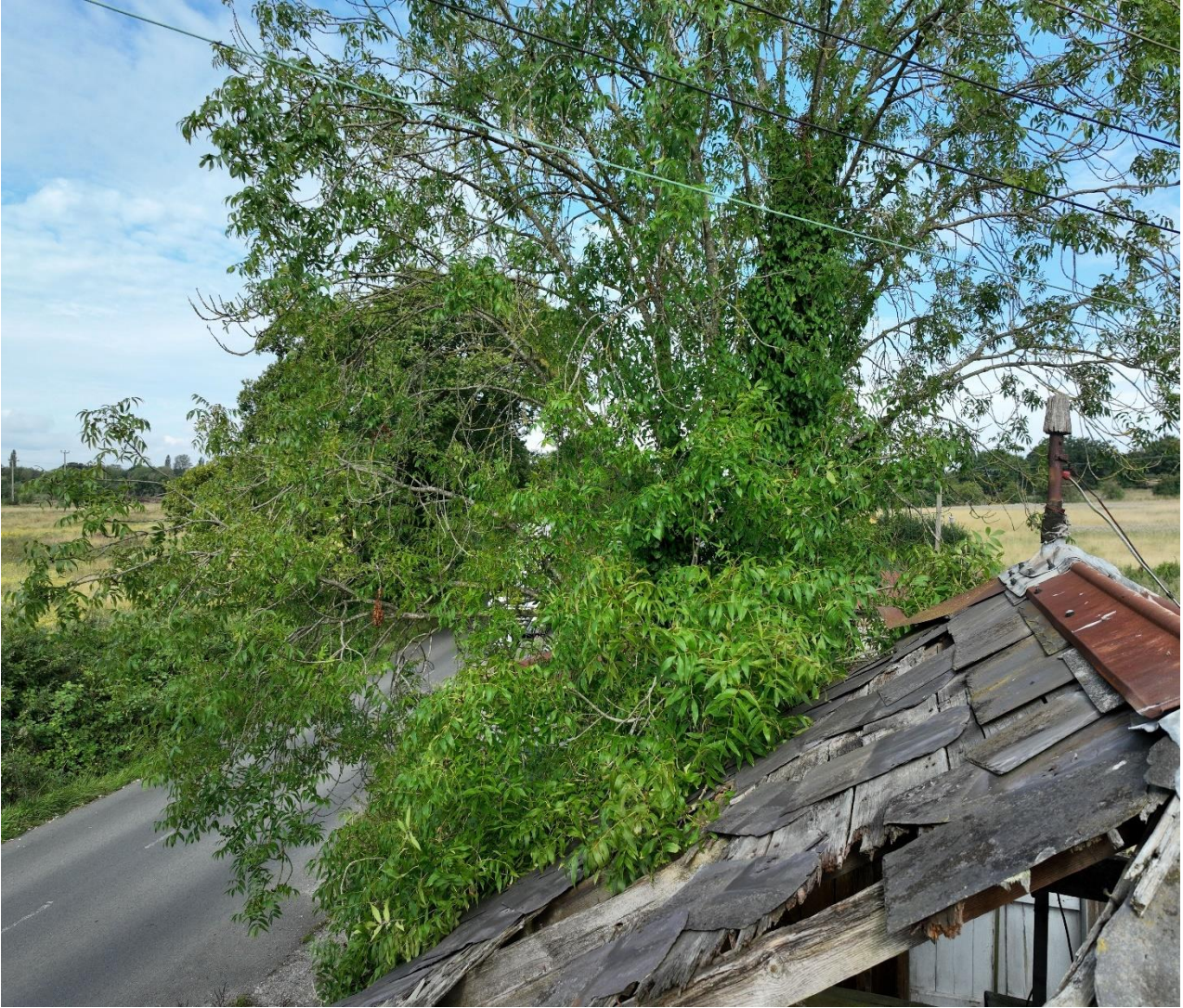
The roof section at W3 is in similar condition to those at the other elevations.
