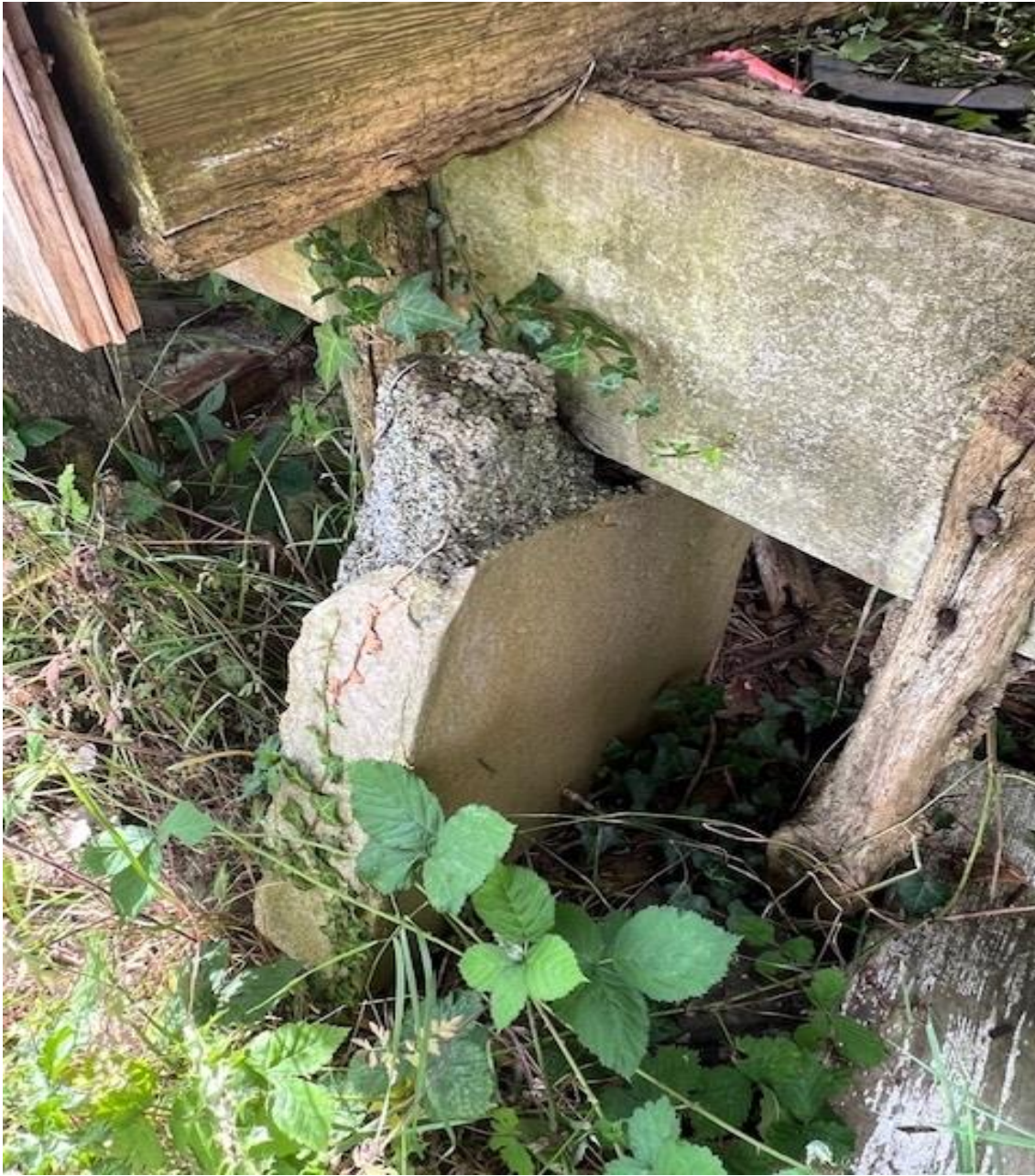
Due to the collapse in areas of the main bearing timbers, here a concrete section has been placed under the main perimeter ring beam timber, to assume add additional support.
