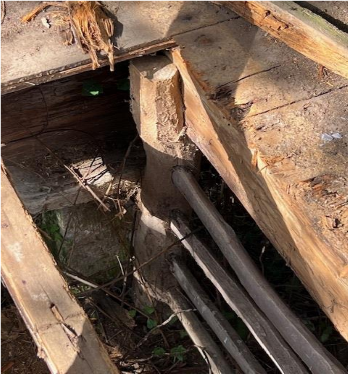
As above, below the main joists there are dividing post and rail timbers.
