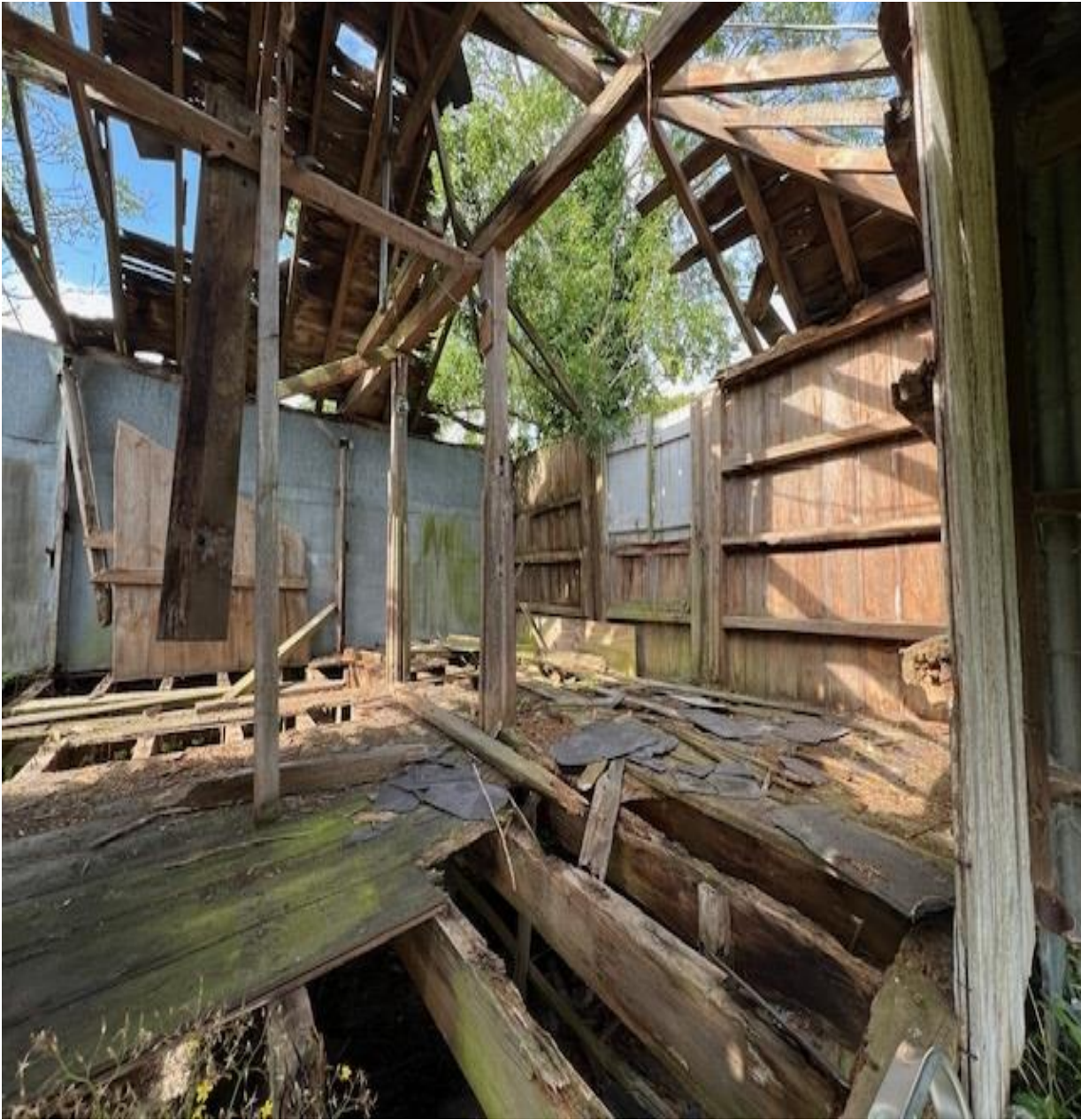
The timber flooring, those at the main bearing joists and the floor boarding laid over all detail significant rot, underfoot they give way.
