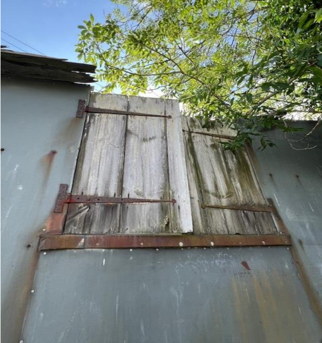
W3 Elevation details two timber shutter doors at the opening – these are hung on metal hinges – which are detailing corrosion.
