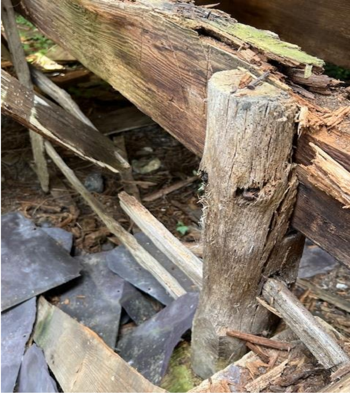
Where the older timber joists sit, and as above there is extensive rot through the full sections of the timber, here the post notched around the timber acting as additional strut support is also decayed, the flight holes detail extensive wood boring insects, the timbers generally detail as wet.
