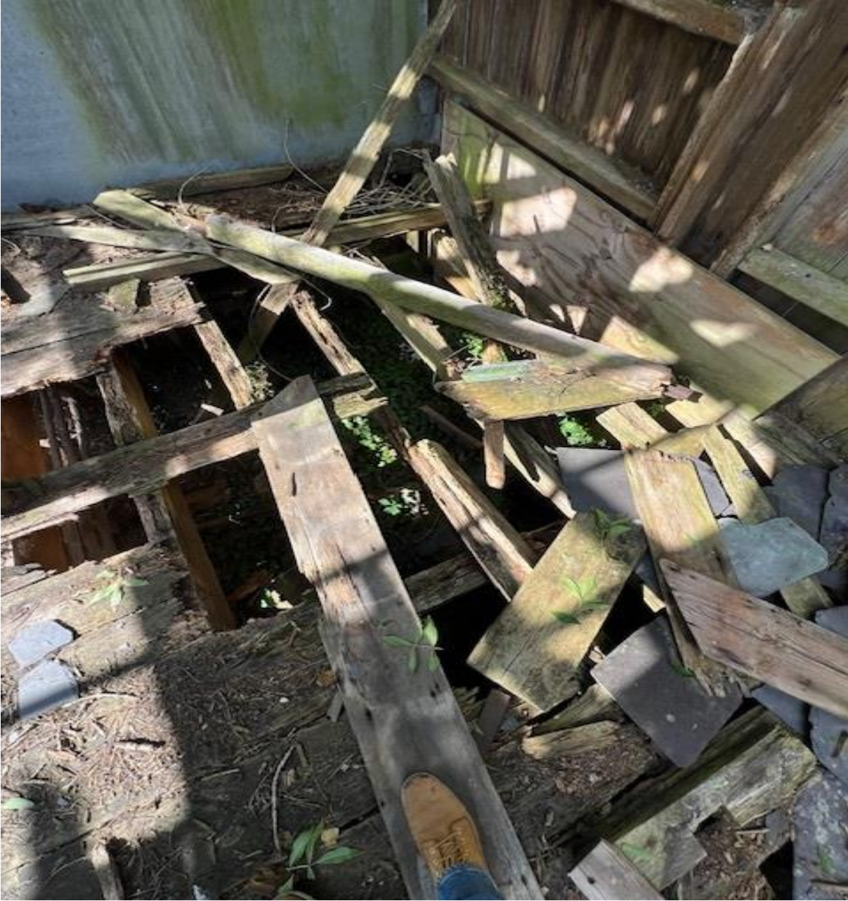
At the corner of the W4/W3 there is little in the way of floor boarding left, the main joists below are decayed to the point that access was restricted.
