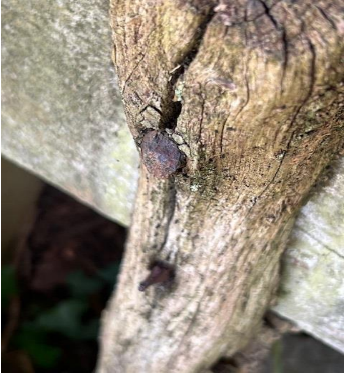
As above, the timber strutting here is nailed to the main 10" x 5" timber.
