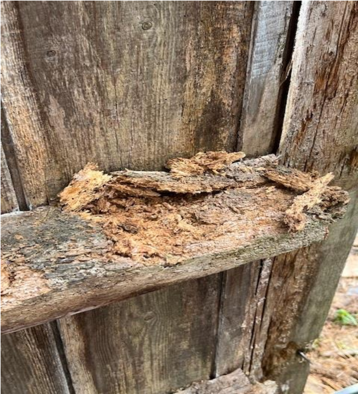
Timber condition of the horizontal brace timber at W1
