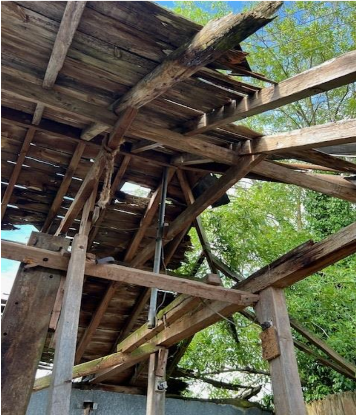
Photos taken from within the building show the extensive decay throughout the roof.
