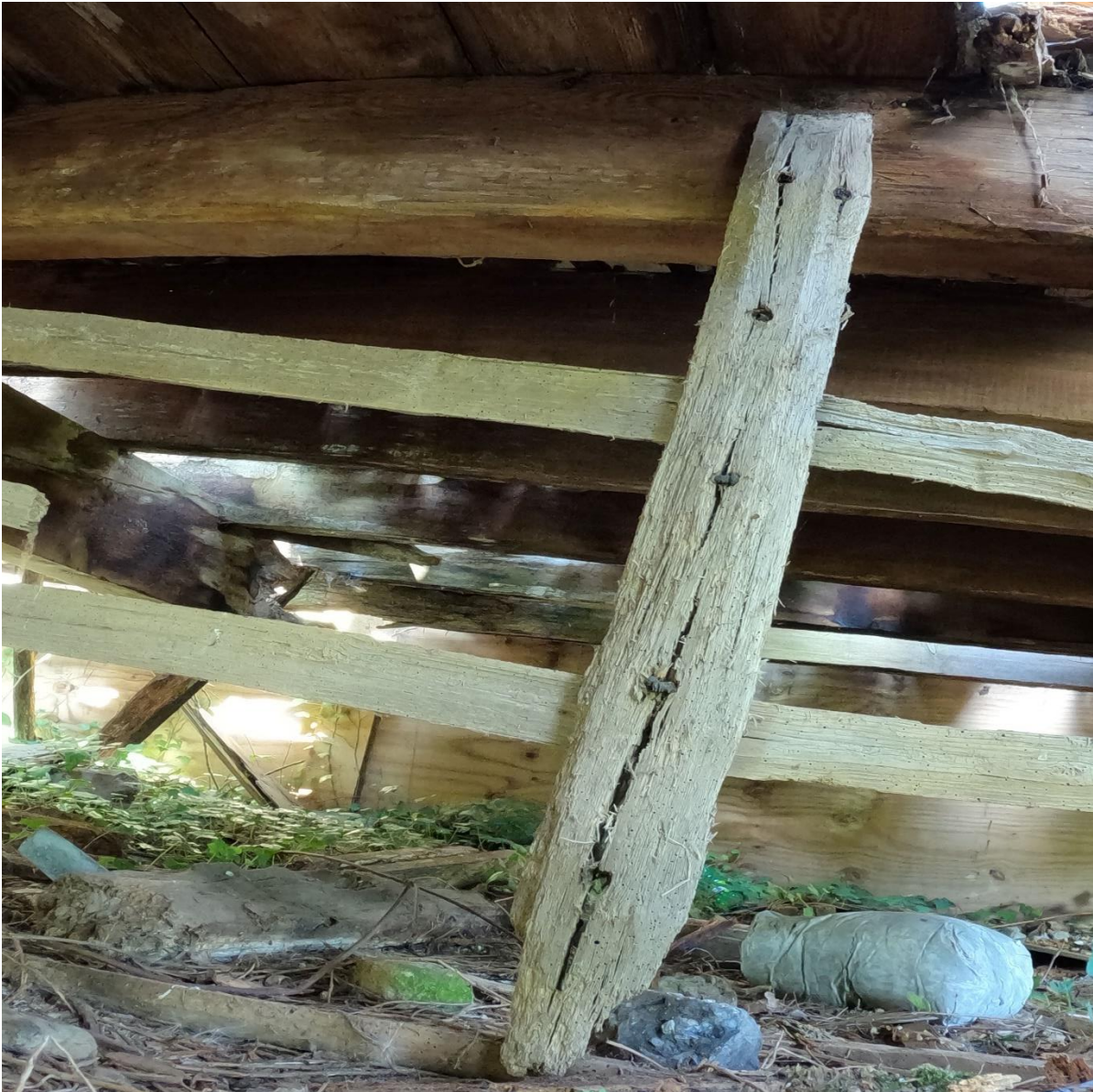
The photo here taken with a pole camera under the main floor shows the underside of the joists to be saturated, and details wet rot and some decay.
