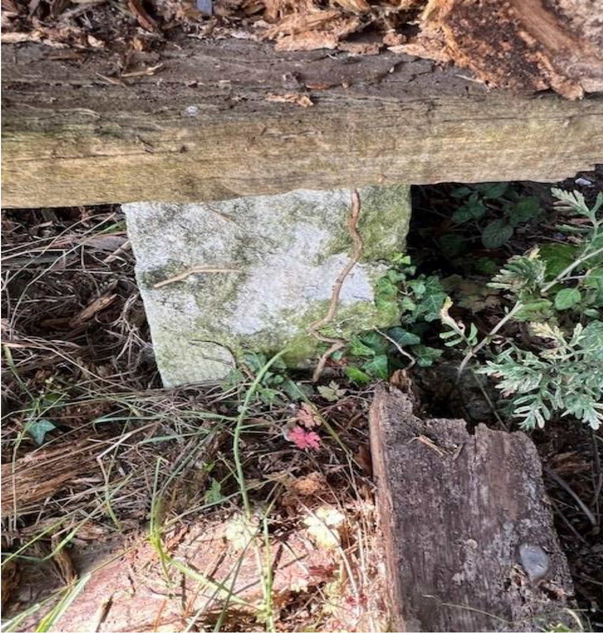
Further example of the staddle stone acting as the support for the main timbers, the stones are in limestone, and although show some sign of decay, the main stone is still structurally supportive.
