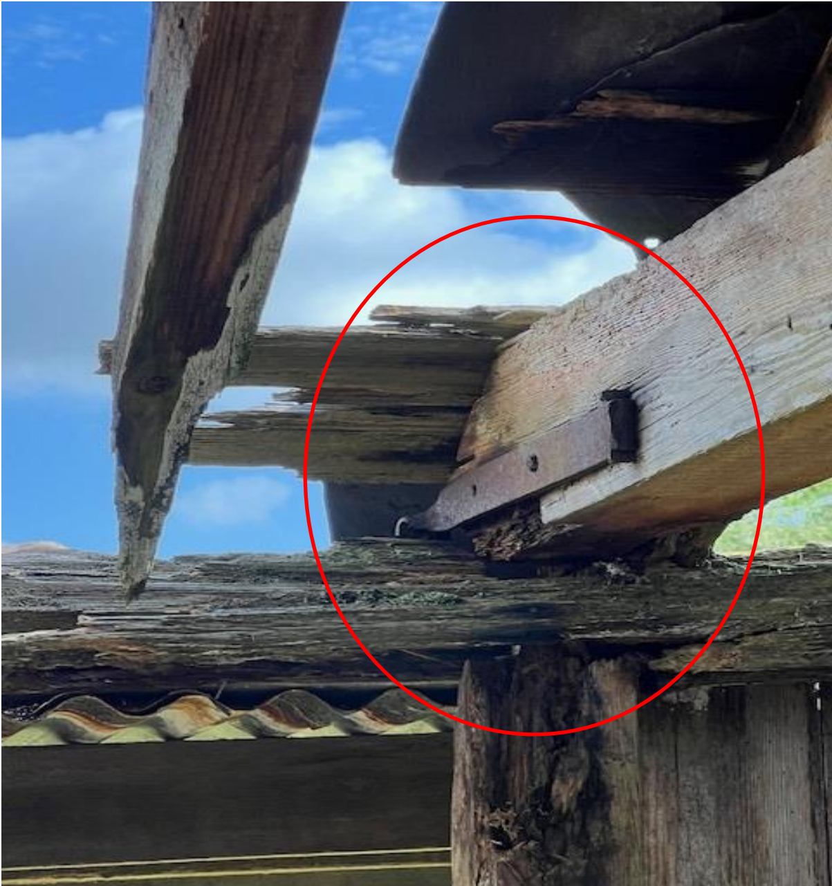
The photo here details the main bearing cross sectional timber sitting on a decayed wall plate, the post below also details extensive decay, the joists ends are no longer in contact with the wall plate in many locations.
