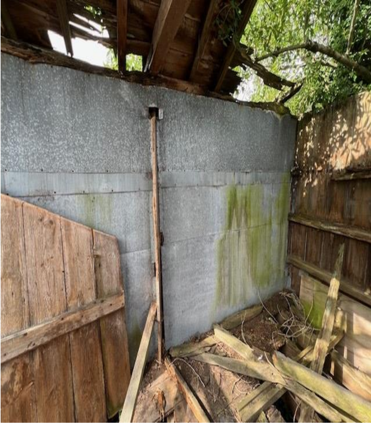
Here the photo details the wall/roof and floor condition at the corner of W3/W4.
