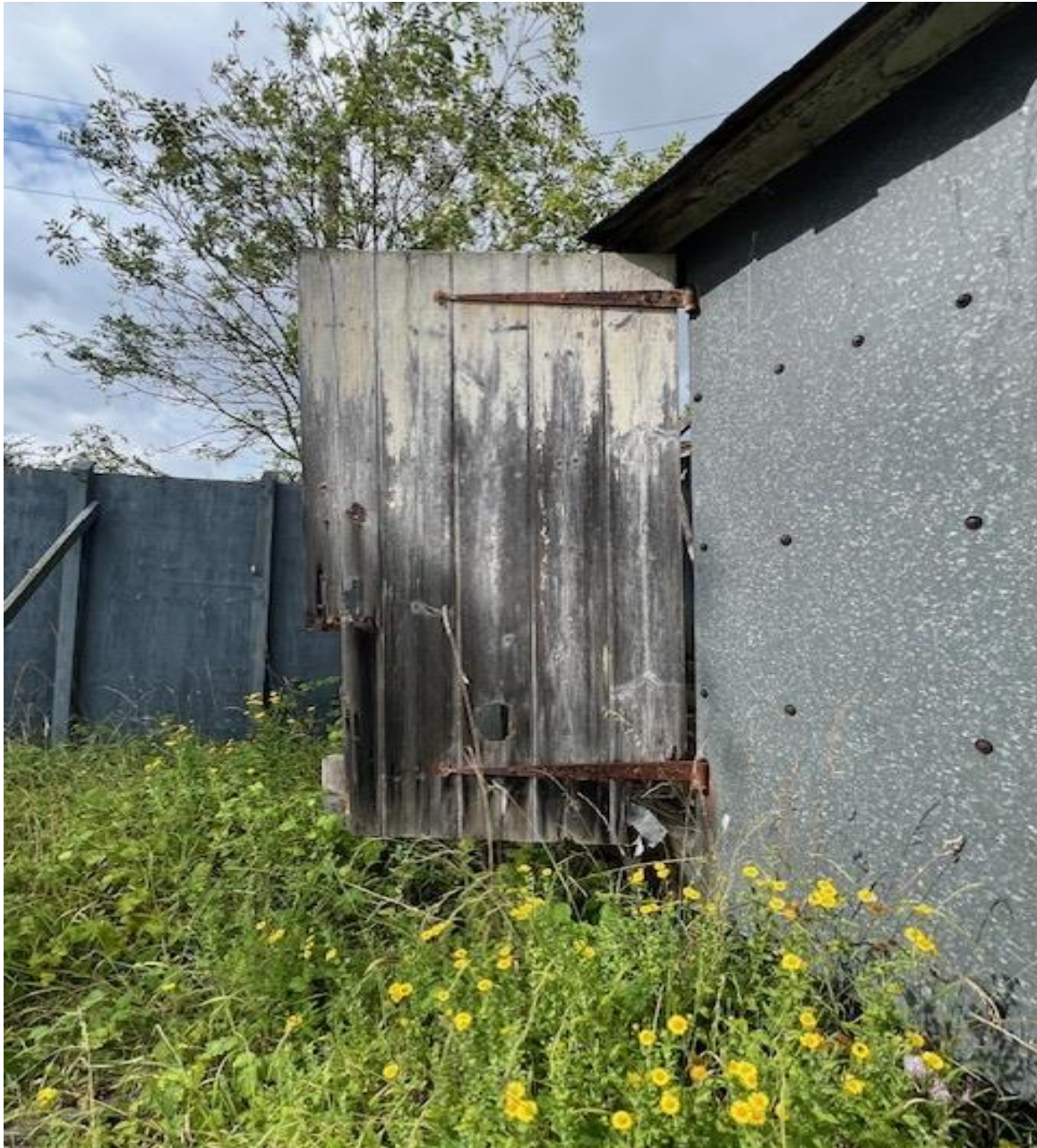
At the W2 elevation, similar as those at W4 there are timber openings with metal hinges, here as opposed to a window, there are double doors, the timbers are again extensively decayed.
