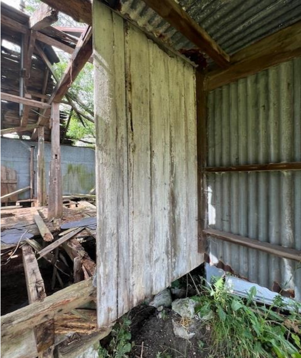
The vertical timbers at W1 have been somewhat protected by the more modern metal canopy and corrugated roofing, but still details as decayed.
