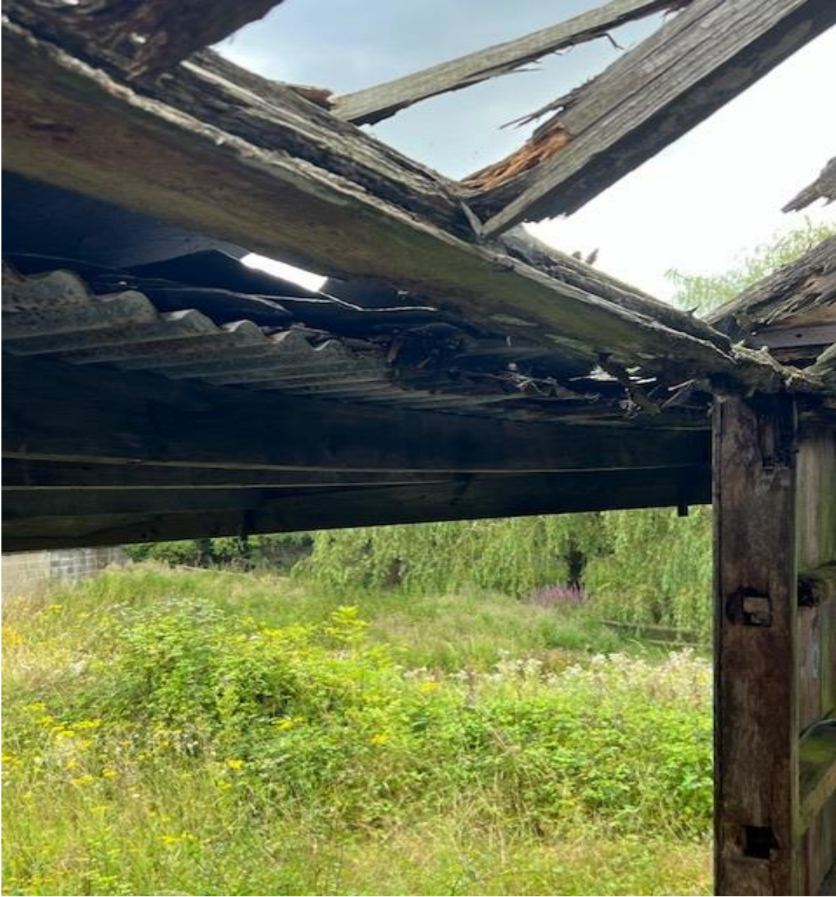
The wall plate which would also be the lintel at the W1 elevation, is decayed to the point of complete rot through the timber.
