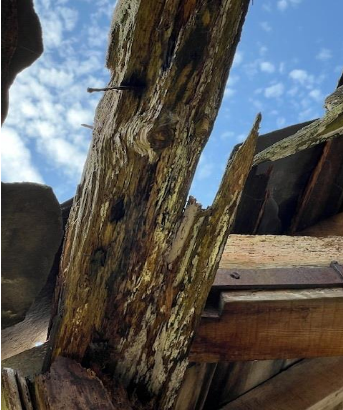
Condition of some of the rafters' still in situ are considered decayed and are suffering from extensive wet rot.
