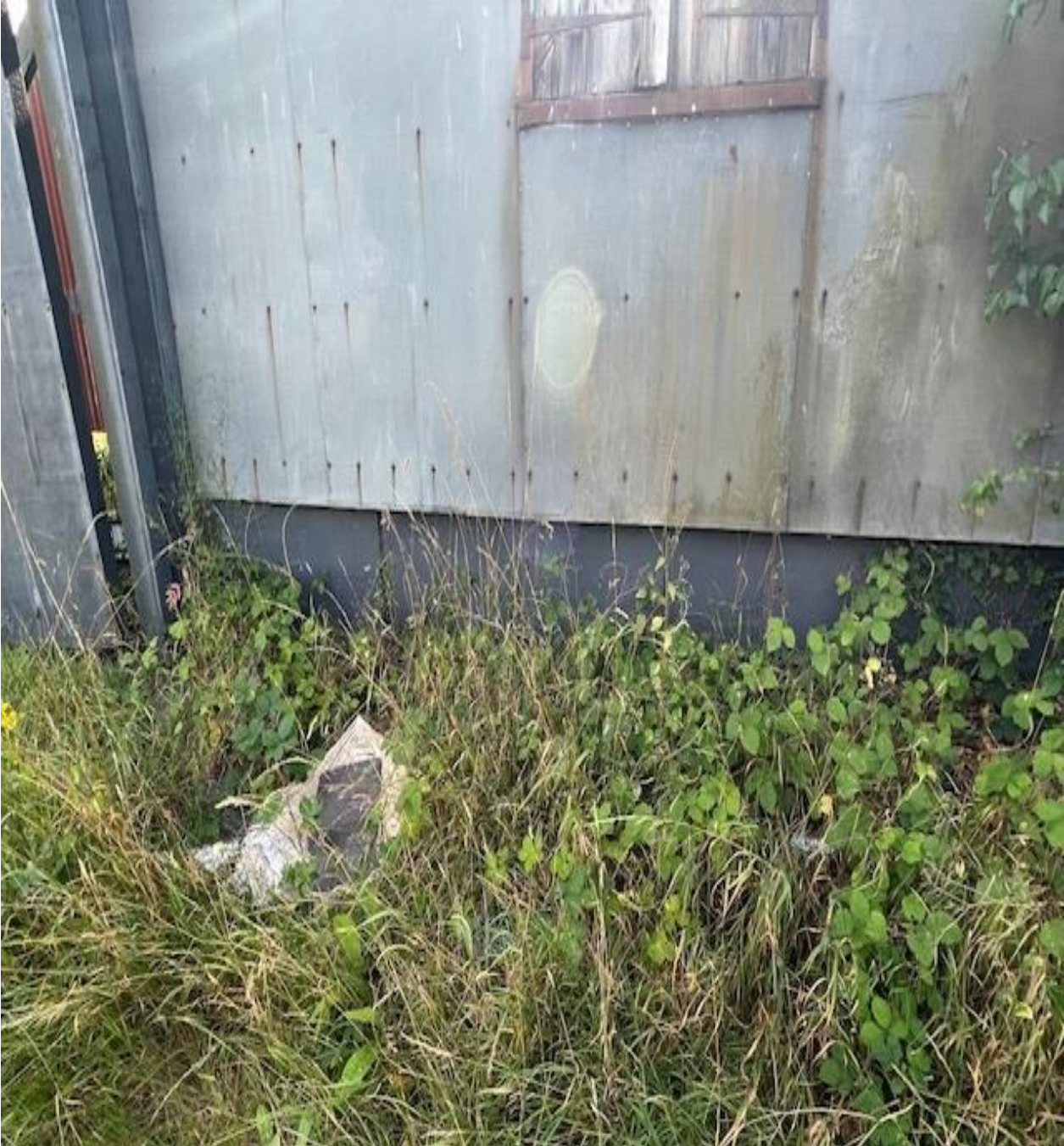
At W3 there is a ply timber base, the main covering at the elevation is cladded in a metal sheeting.
