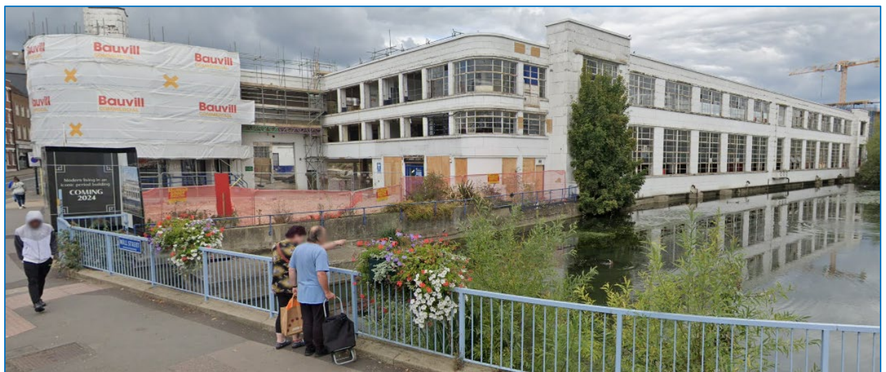
Figure 12: Len House, Maidstone Town Centre (site allocation LPRSA145) (image: Google Maps, Sept 2022)
