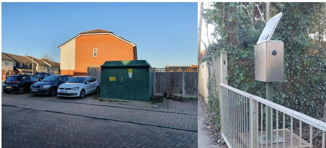
Figure 32: A bad and good example of integrating and visually screening utility infrastructure and equipment – the Hardwicks and Ulcombe Road
