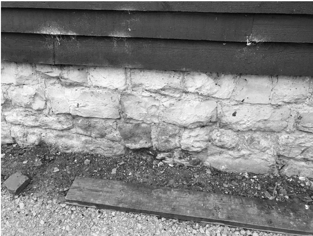
Rising damp evident within the Kentish ragstone random wall plinth.
