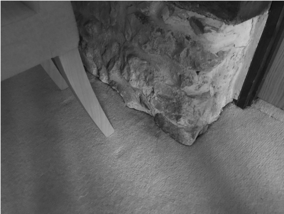
Mould and damp below moquette of living room on the ground floor
