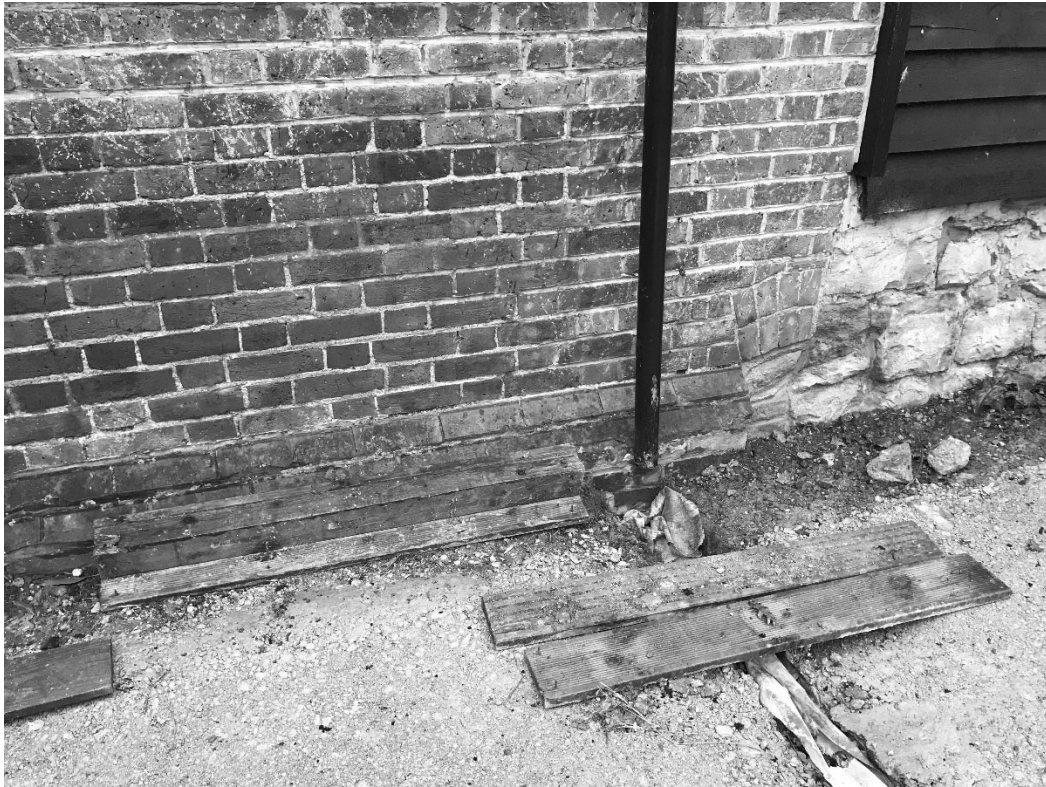
Recent repair of saturated stonework to plinth on north side of the Barn and rising damp within brickwork to left
