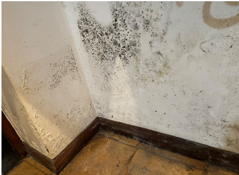
Damp within the property
