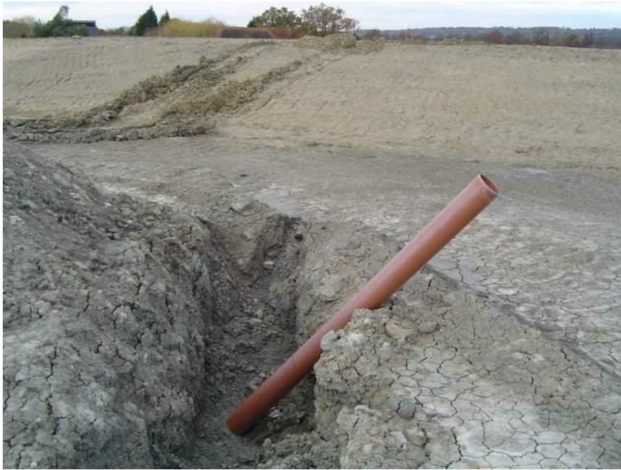
Close-up of outlet pipe
