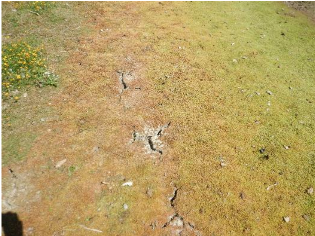
Photograph 8 Desiccation cracking in clay
