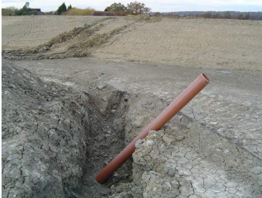
Close-up of outlet pipe
