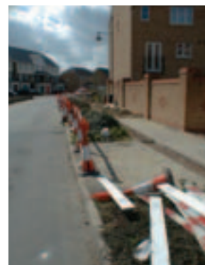
Above, where existing paving is disturbed to allow for the installation of services it should be reinstated with the original or closely matching materials, particularly in the case of traditional brick, stone, stone setts and cobblestone pavings.
