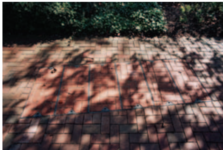
Top, a manhole cover showing how paving can run across the top within a recessed cover.
